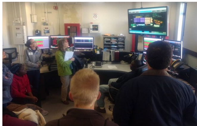
Participants tour the control room from which employees can monitor and control plant operations.
